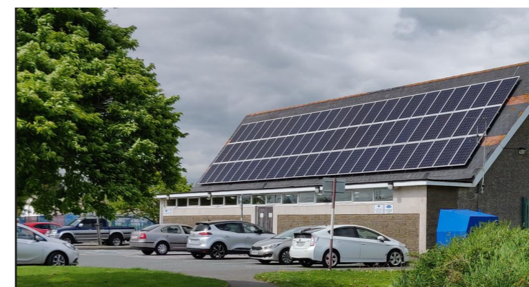
Solar PV rooftop array at Arklow's Coral Leisure Centre and Pool
